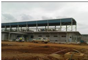
C2 – Operation Control Room
